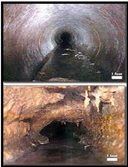
Bottom View: Actual photo by remote control camera of a grease clogged sewer pipe
