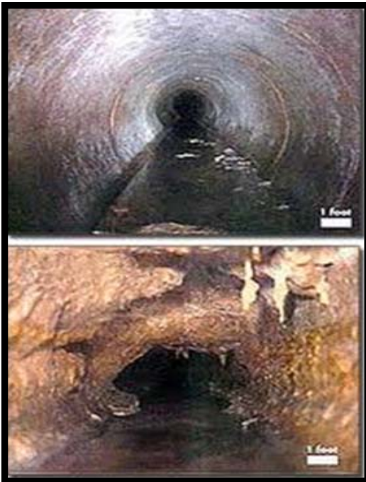
Bottom View: Actual photo by remote control camera of a grease clogged sewer pipe
